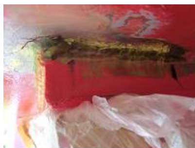
Fig. 3 The welding section crack-generations were recognized.
