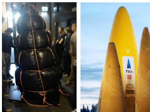
Fig. 3 Inflatable formwork. Left: Scale model test. Right: about 30 m high main tower (back) and about 22 m high front towers (photo: Bart van Overbeeke, TU/e)
