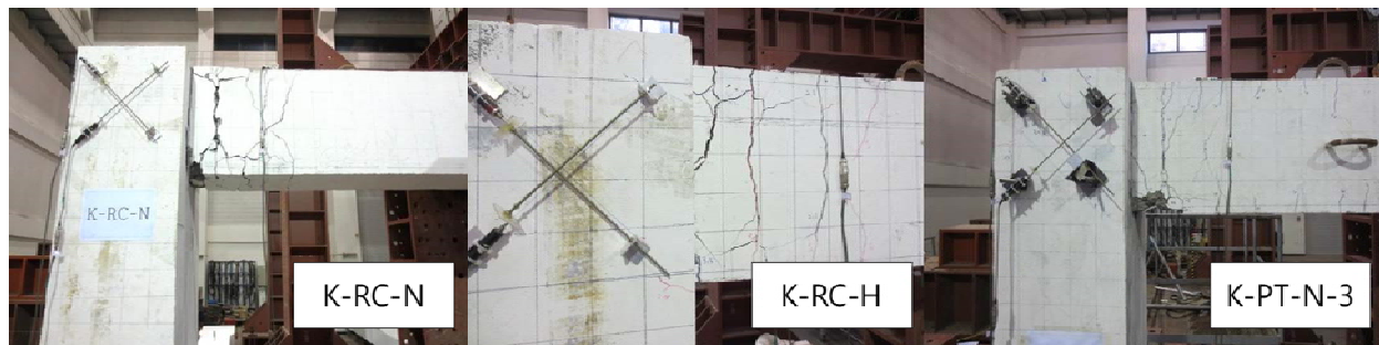
Fig. 6 Final crack patterns
