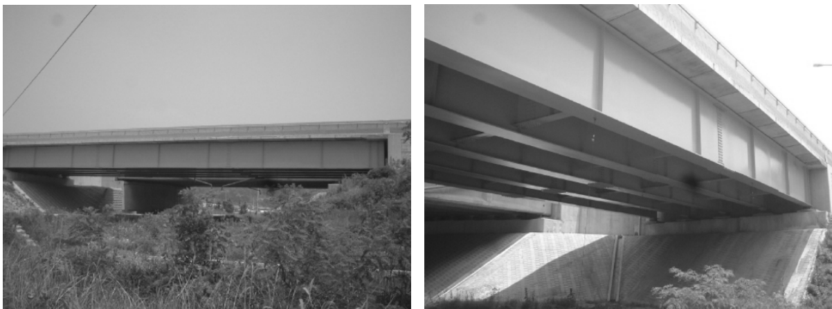
Fig. 1 Front view (left) and bottom view (right) of Samseung Bridge (Yi et al. 2007)
