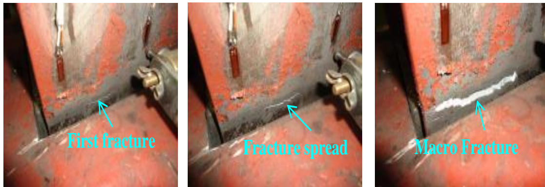
Figure 8. Step-by-step spread of fracture throughout the pile flange.
