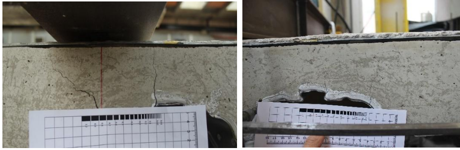
Fig. 13 Concrete cracking at and between loading points (B1b)
