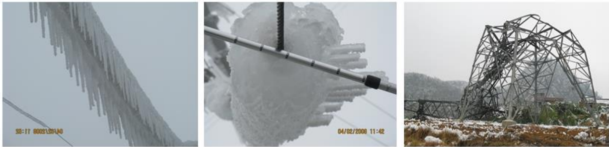
Fig. 1 Ice disaster in transmission towers
