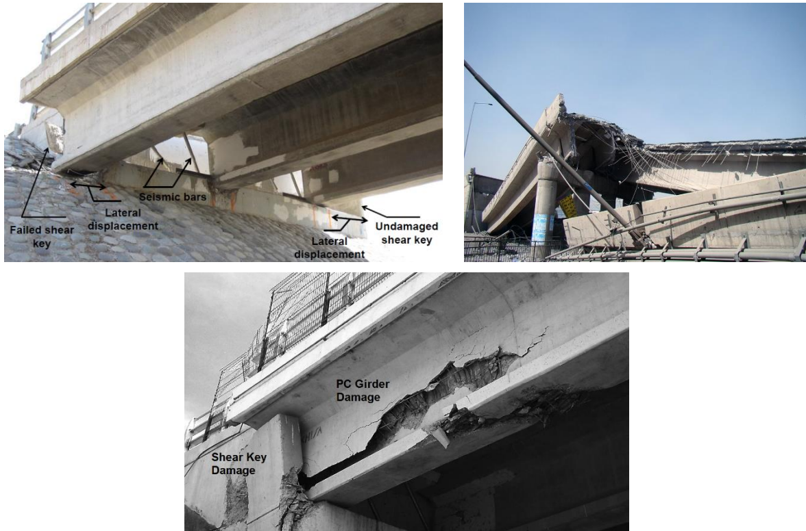
Fig. 1 Damage observed in highway bridges after the 2010 Maule earthquake. (Photos: M. Yashinsky, J.L. Seguel, F. Schanack)
